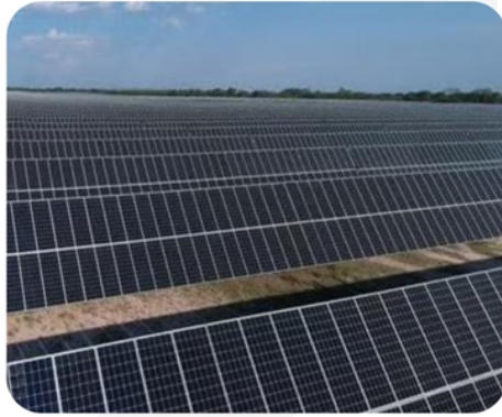
Teraco will own and wheel power from a 120MW solar plant to sustainably power its data centers for cloud and AI computing
