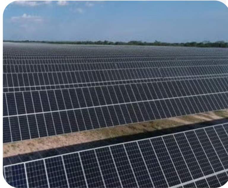
Teraco will own and wheel power from a 120MW solar plant to sustainably power its data centers for cloud and AI computing
